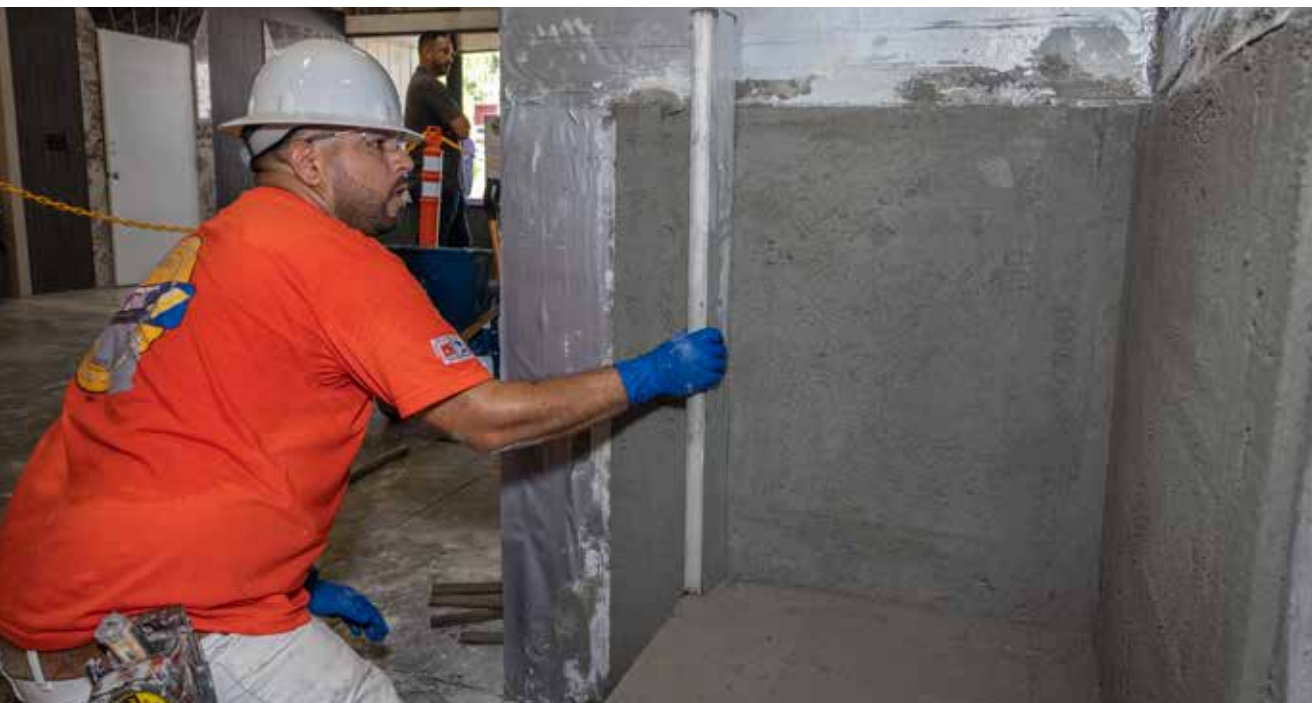
Apprentice Arturo Flores of BAC Local 4 took second place in Tile. Here, he checks his work on a shower enclosure.
