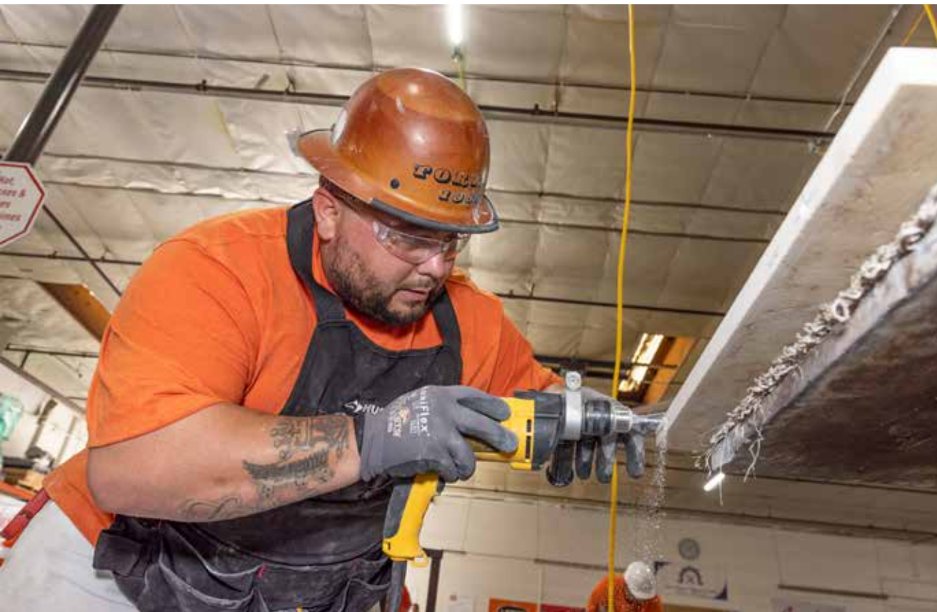
BAC Local 4 Marble Mason apprentice Joseph Torres drills holes for a “spot and anchor” installation of a marble panel.
